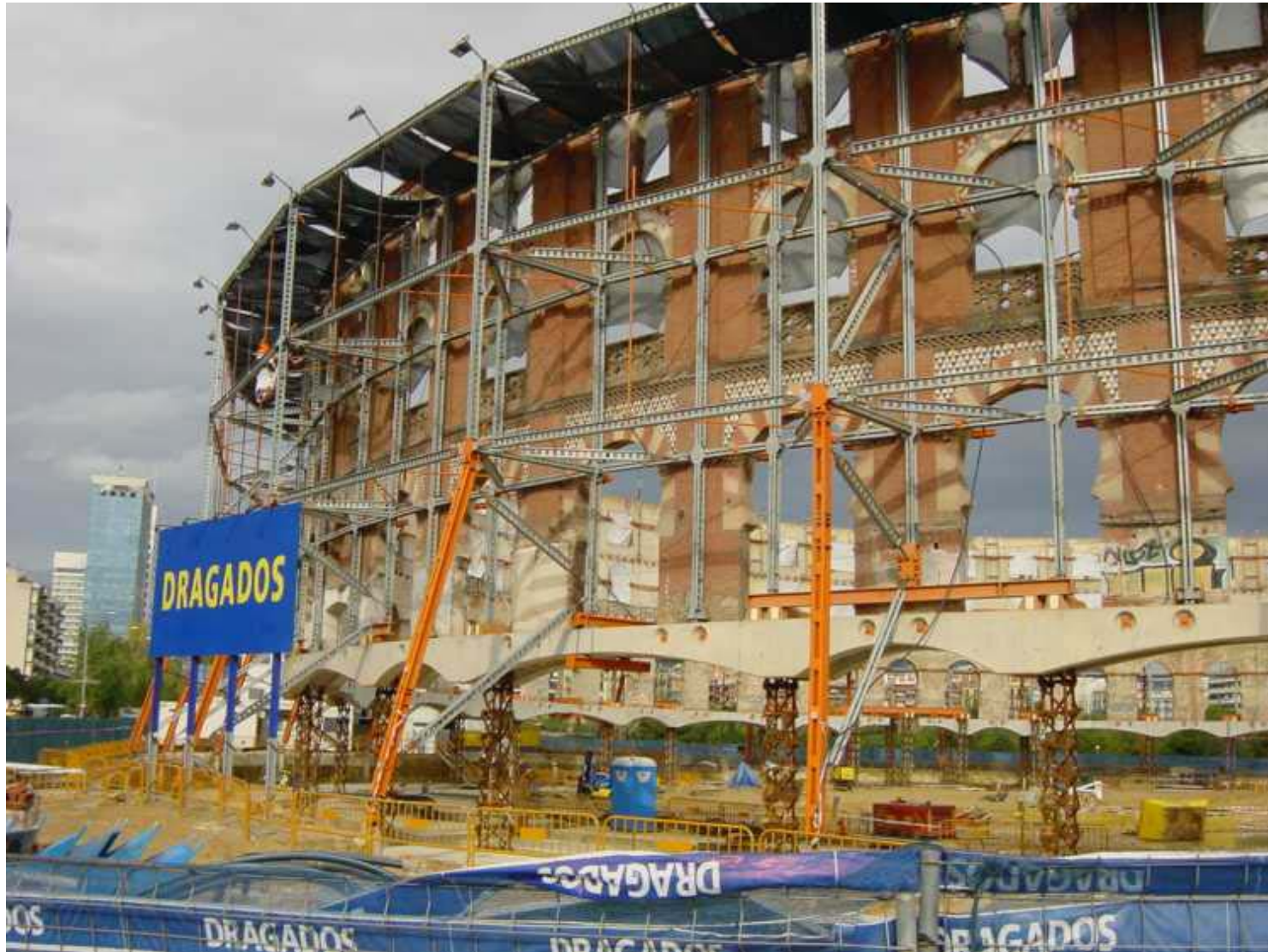
Free standing facade of bullring, supported by micropiles and braced by framework. Beginning of excavation.
