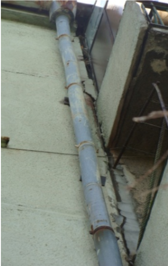
Picture 1: Vertical joints opening between façade panels
