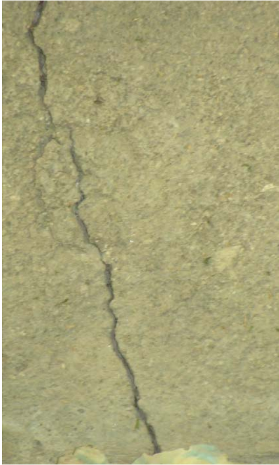
Picture 3: Cracks in the foundations
