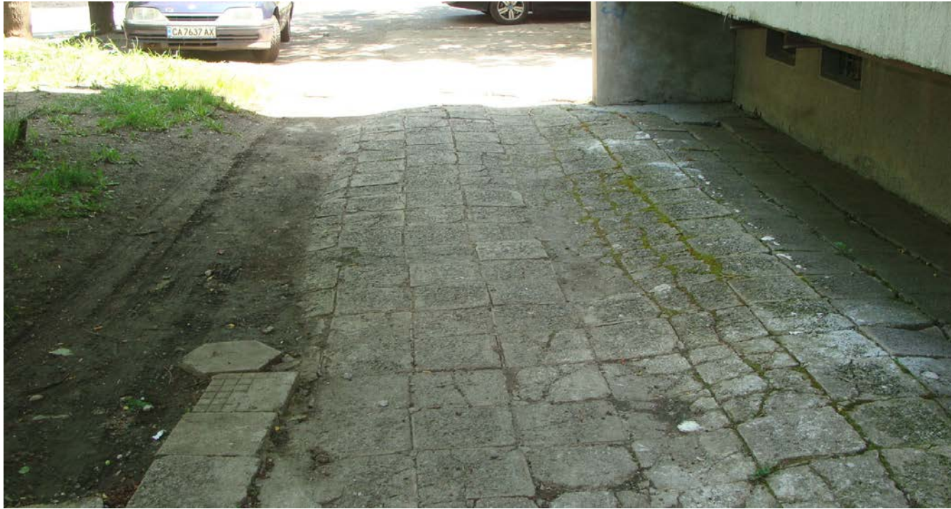
Picture 4: Broken sidewalk pavement around section A
