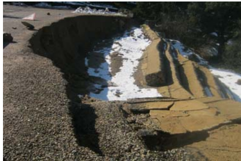
Photo 1: Old landslide reactivated, previously stabilized by a flexible gabions wall
