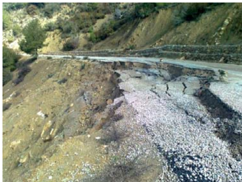
Photo 3: Landslide: failure occurred
