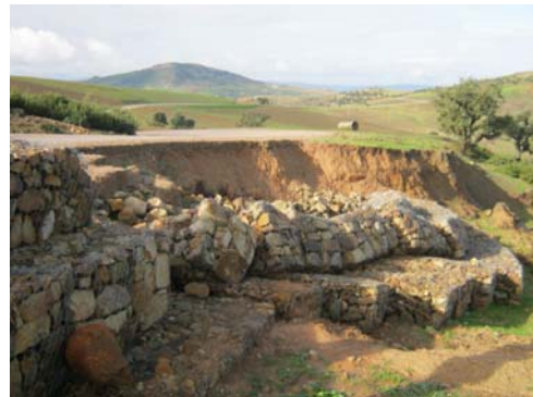
Photo 4: Old landslide reactivated previously stabilized by gabions wall
