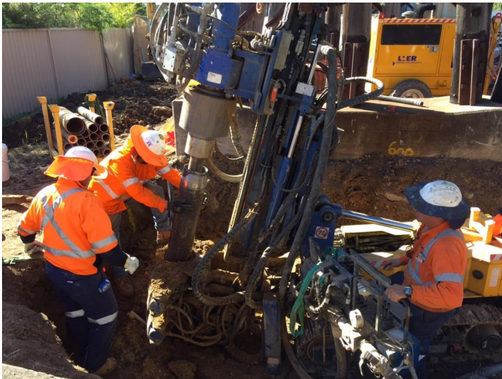
Figure 4: Common Drilling Practice in Australia – E-Stops and Trip Wires
