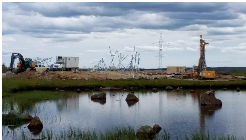
Figure 7. Boggy/wet ground conditions
